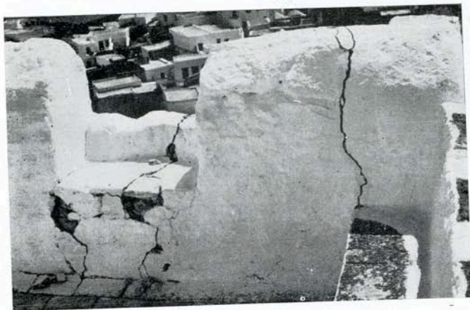
Fig. 26 —Cracks on the wall-fence of the building of Patmos Island Monastery caused during the earthquakes of July 9, 1956.
