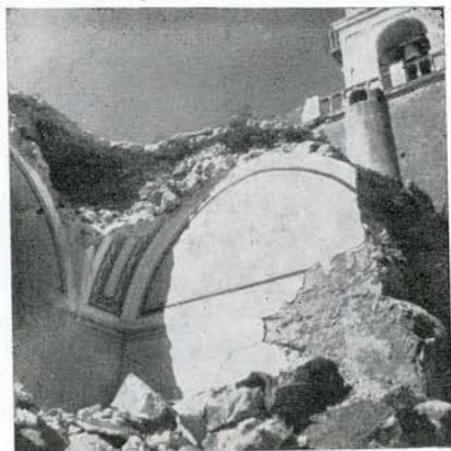
Fig. 18 —The inner side of Anastasis Church in Hemerovigli showing the poor construction, after the earthquakes of July 9, 1956.
