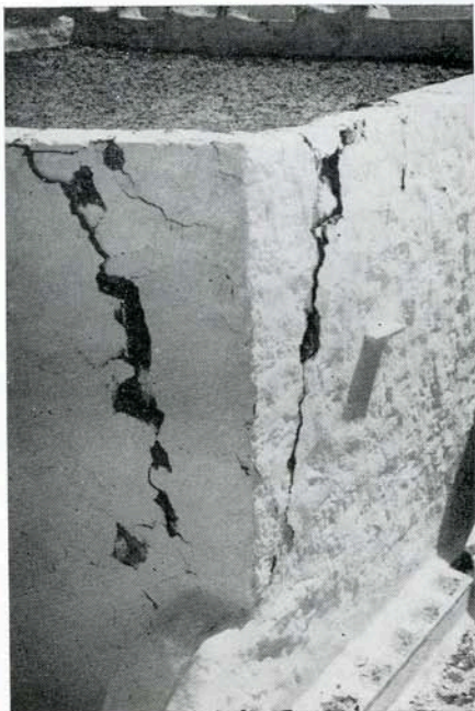
Fig. 24 —Another view of the heavy cracks made to the building of Patmos Island Monastery by the earthquakes of July 9, 1956.
