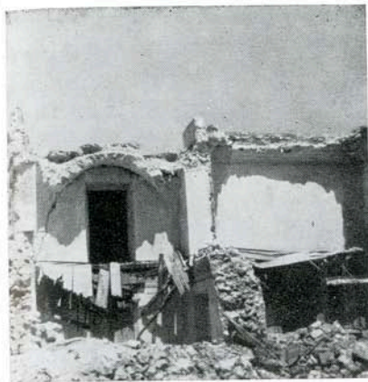
Fig. 11 —Failure of vaultings of different construction in Phira, during the earthquakes of July 9, 1956.
