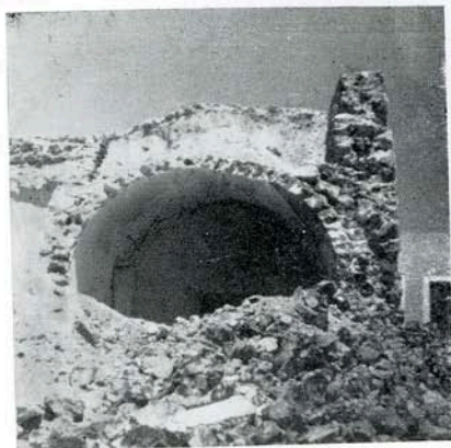
Fig. 12 —A view showing the poor construction of the heavy vaultings in Phira, after the earthquakes of July 9, 1956.
