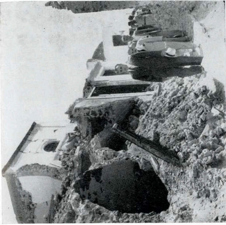
Fig. 6 —Tunnels underlying the houses in Phira, Thera Island, after the earthquakes of July 9, 1956.
