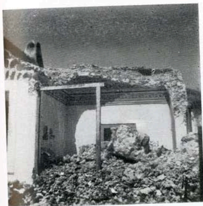
Fig. 21 —Destruction of houses with heavy roof in Messaria by the earthquakes of July 9, 1956.
