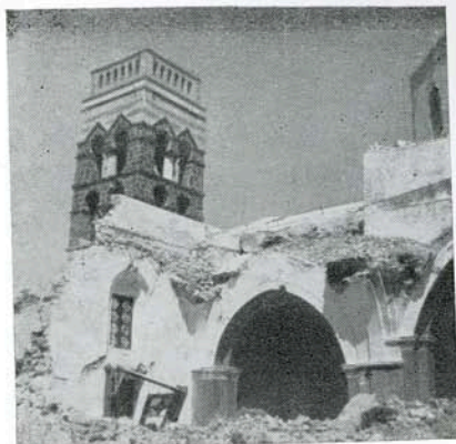
Fig. 16 —The bell tower of Malteza Church in Hemerovigli left intact by the earthquakes of July 9, 1956.
