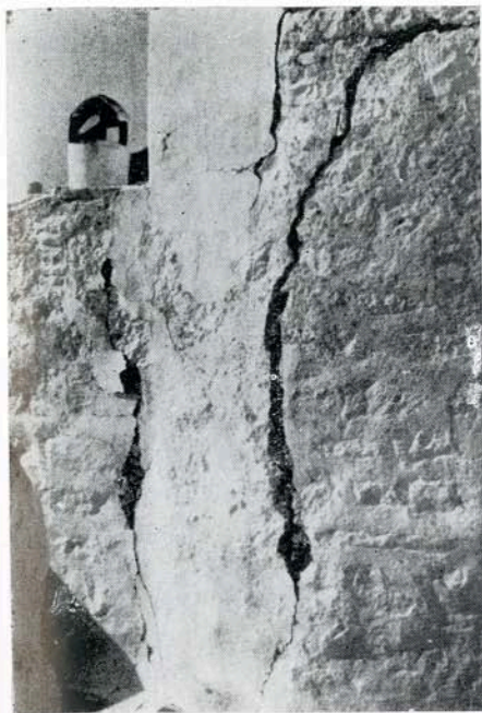
Fig. 23 —The building of Patmos Island Monastery was heavily cracked by the earthquakes of July 9, 1956.
