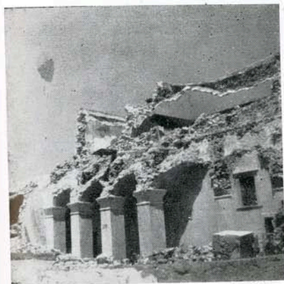
Fig. 13 —A building with a very heavy roof in Phira, ruined by the earthquakes of July 9, 1956.
