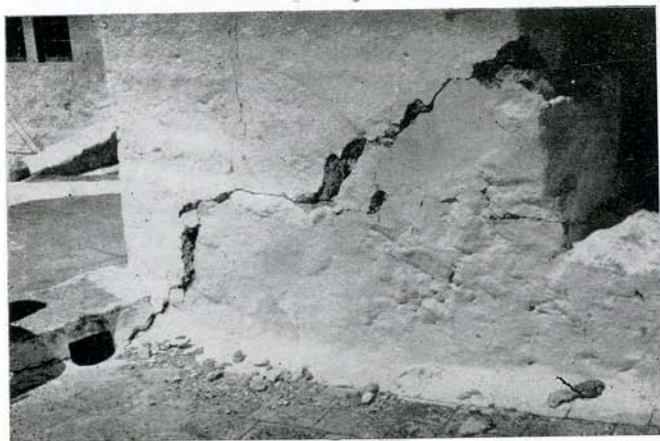
Fig. 25 —Another view of the badly damaged building of Patmos Island Monastery by the earthquakes of July 9, 1956.
