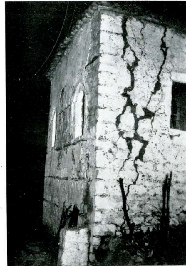
Fig. 1.—A sight of the earthquake failure in Grekochori after the shock of February 4, 1958. Note the very poor construction of the house.
